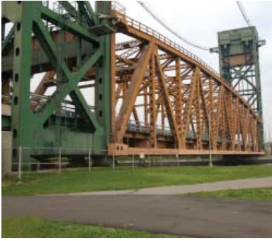
In 2006 Hamilton and Burlington completed a project to improve trail use crossing the boundary over the Lift Bridge. Formerly this involved a dangerous road crossing. Today, trail traffic is routed under the bridge away from vehicular traffic. The local cycling committee is pursuing the idea of installing a cantilevered addition to the lake-side of the bridge for cyclists. Source: Simon Wilson
