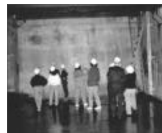
Solutions for combined sewer overflows will likely include a combination of structural techniques - such as the Eastern Beaches detention tanks, seen here from the inside prior to operation - and non-structural techniques.
